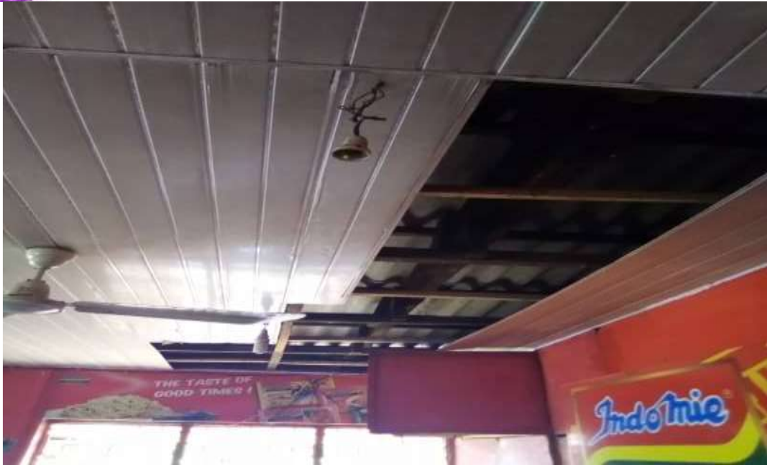
Figure 2: Collapsing PVC ceiling in Hall 3 Common Room
