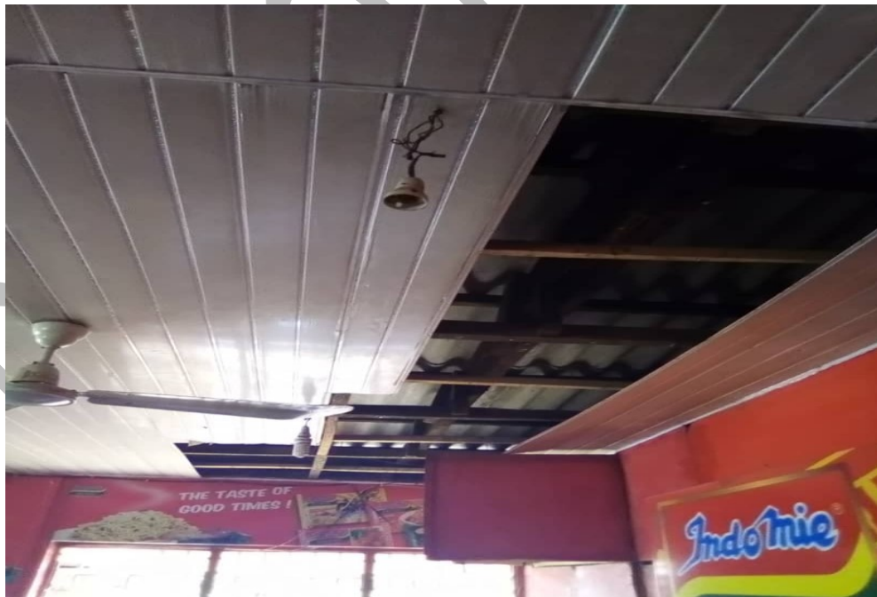
Figure 2: Collapsing PVC ceiling in Hall 3 Common Room
